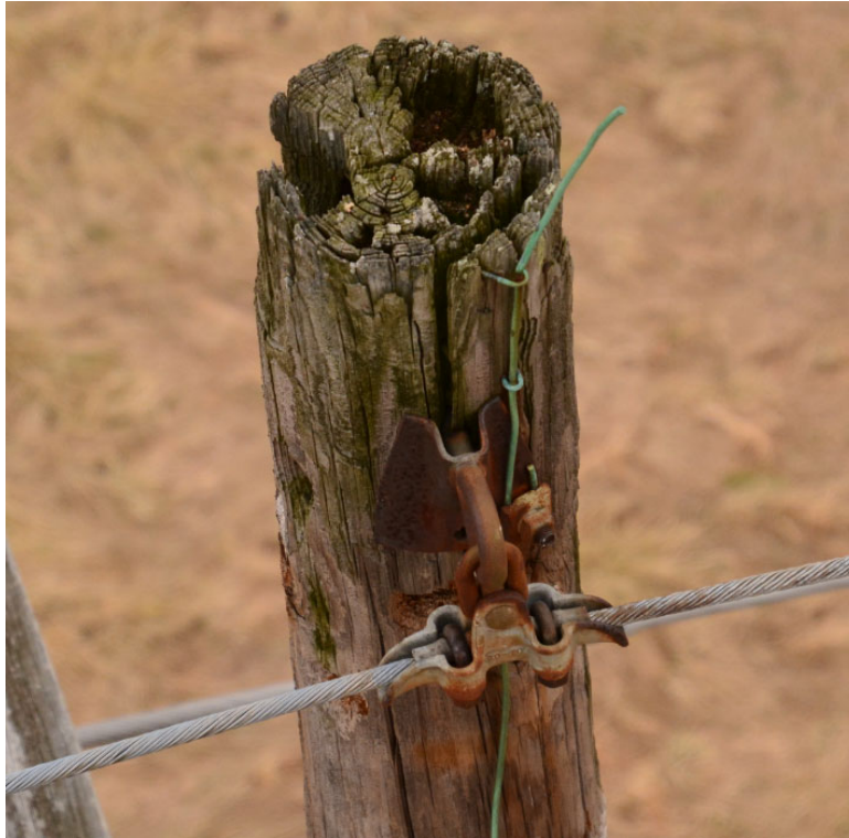
Photograph 3: Pole top rot and woodpecker damage
