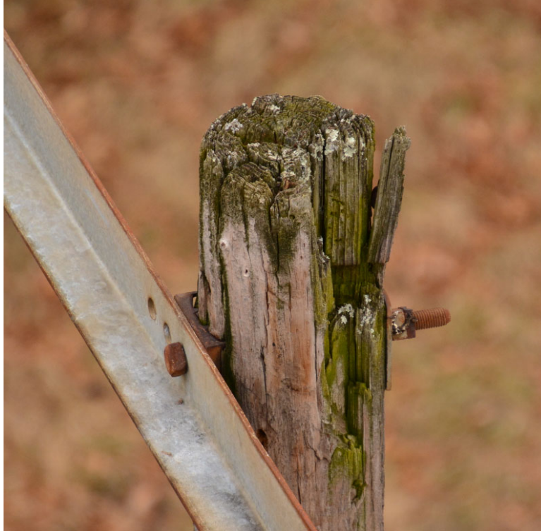
Photograph 1: Pole top rot (common on majority of wood poles on the Line)
