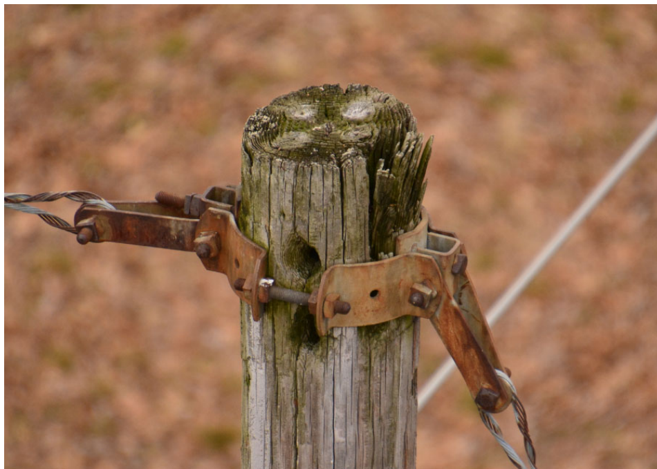
Photograph 2: Pole top rot and woodpecker damage
