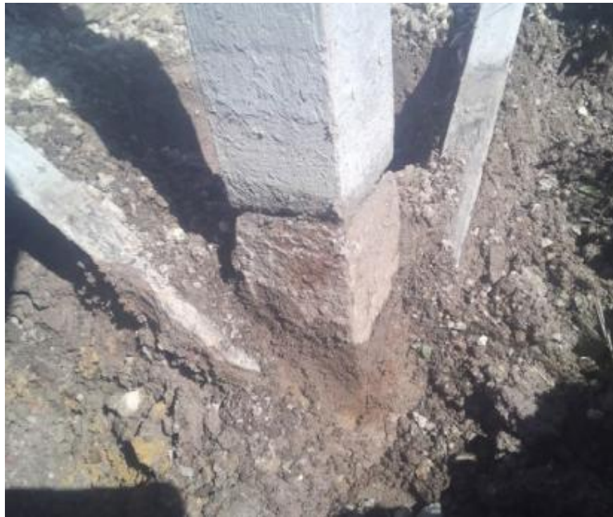
Photo 2. Priority 1 condition on leg 3 of tower 6699.
