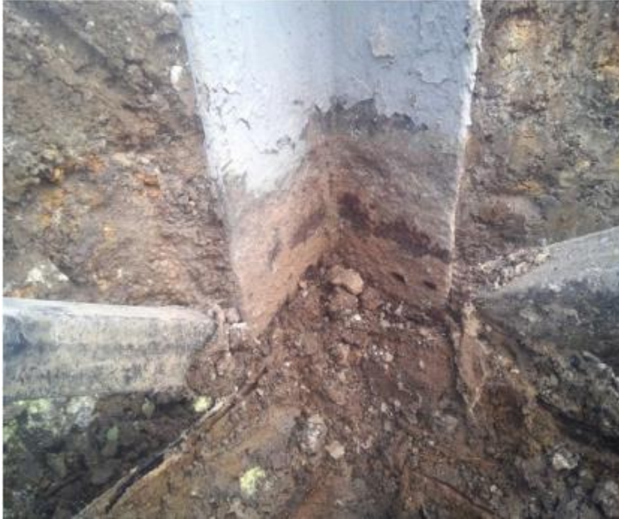
Photo 1. Priority 1 condition on leg 1 of tower 6699.
