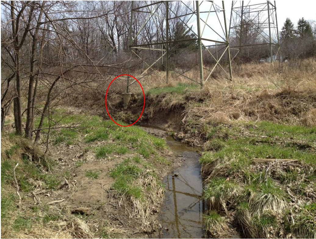
Photo 1. Tower 2047 and adjacent creek. The exposed tower leg is circled in red.
