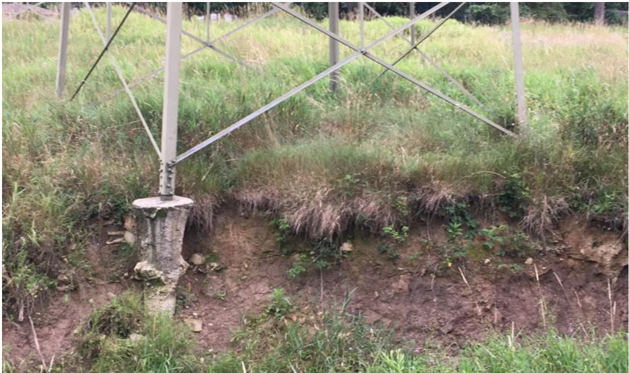
Photo 2. Erosion near two tower legs.
